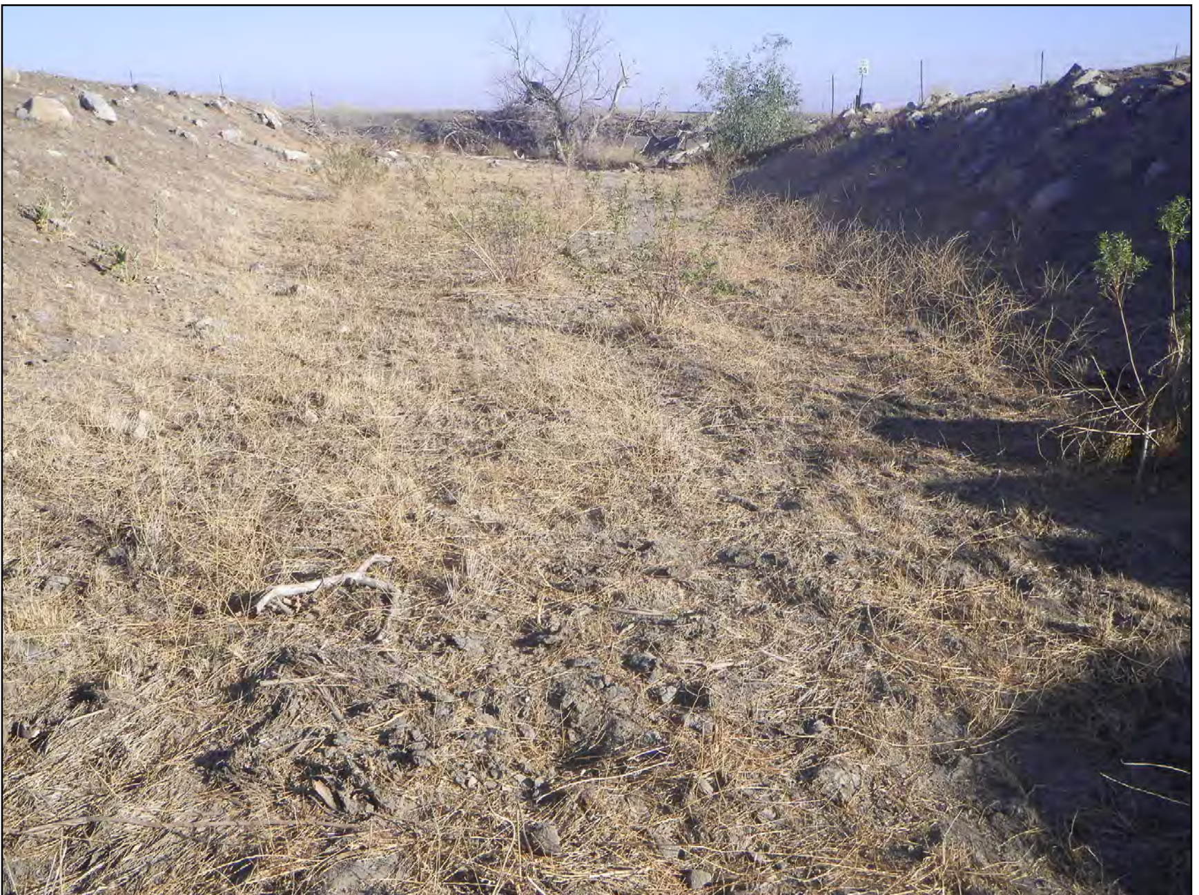
BELOW: Photo 10. Representative view of Impact Area at Live Oak Creek Drainage; Conditional Assessment Area GV-AA10 (October 10, 2014)
