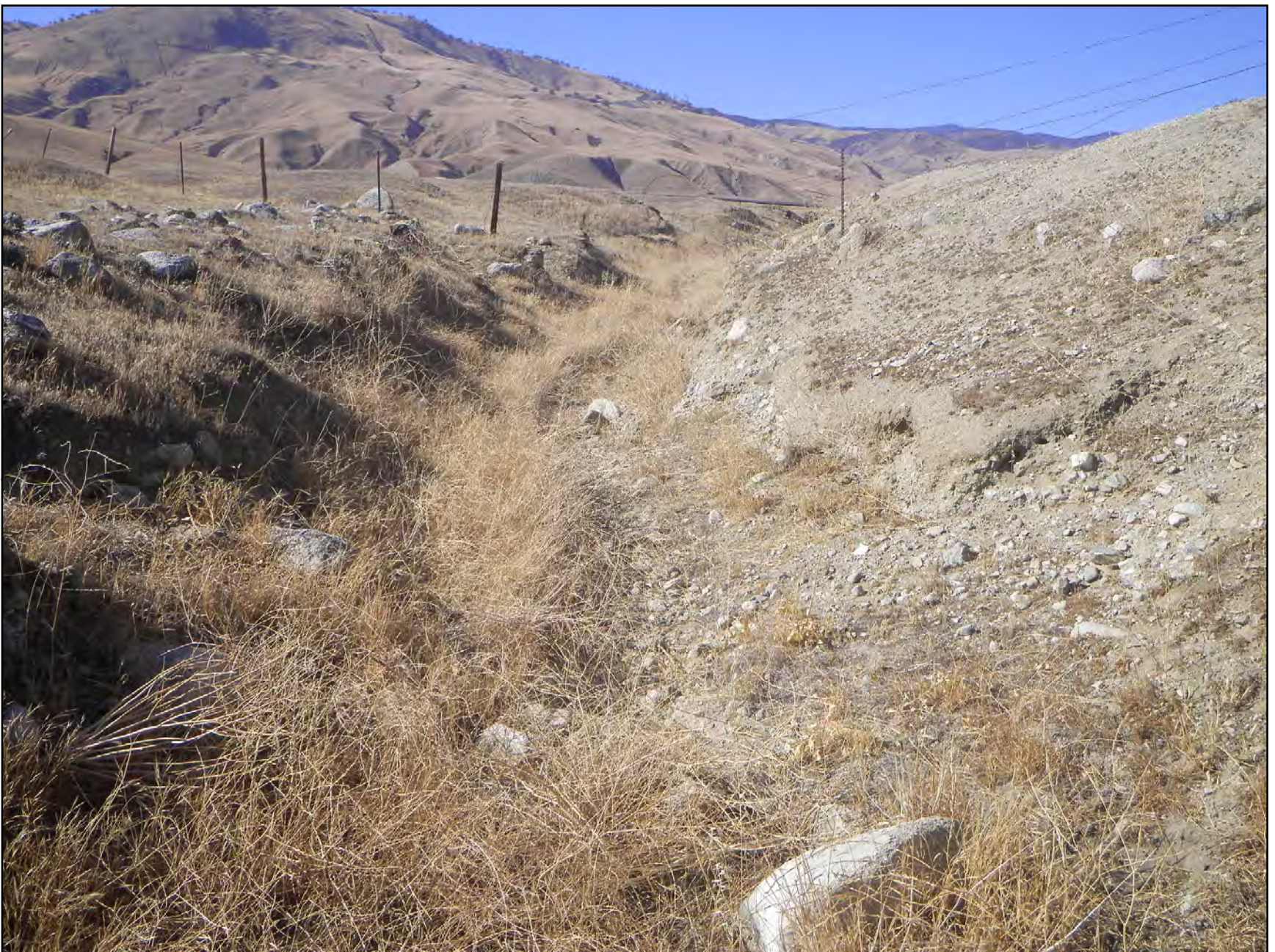
BELOW: Photo 8. Representative view of Impact Area at Cattle Creek Drainage Downstream; Conditional Assessment Area GV-AA8 (October 10, 2014)
