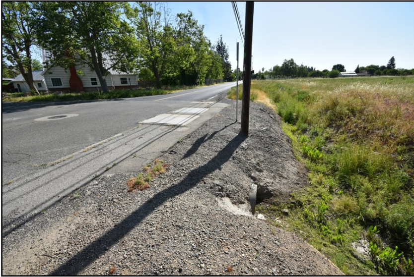
Photo 1: Ditch along south side of Little Avenue, looking east along paved road work area.
