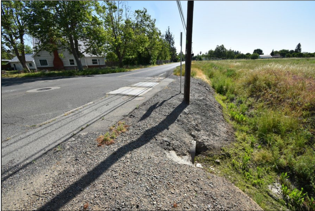
Figure 7. RD-01. Ditch along south side of Little Avenue, looking east along paved road work area
