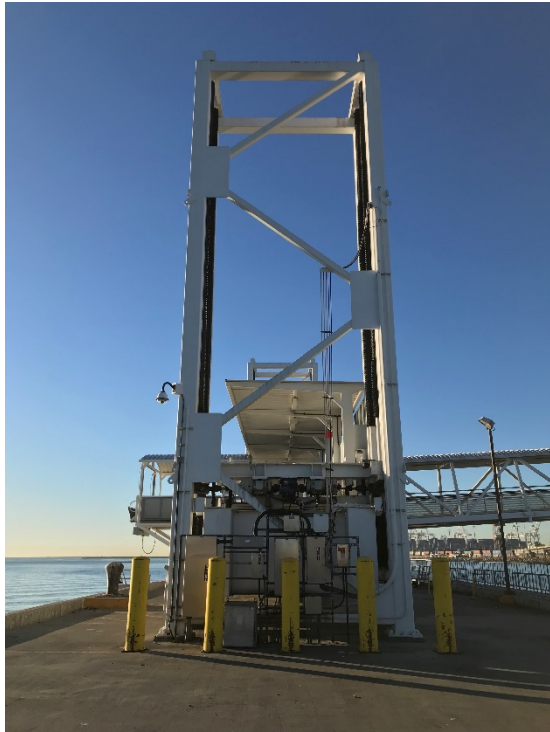
Photo 11 - Passenger bridge lift system
