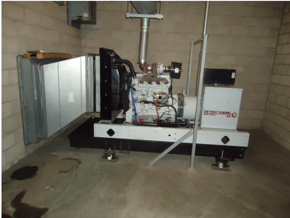
Photo 22 - Diesel-powered emergency generator
