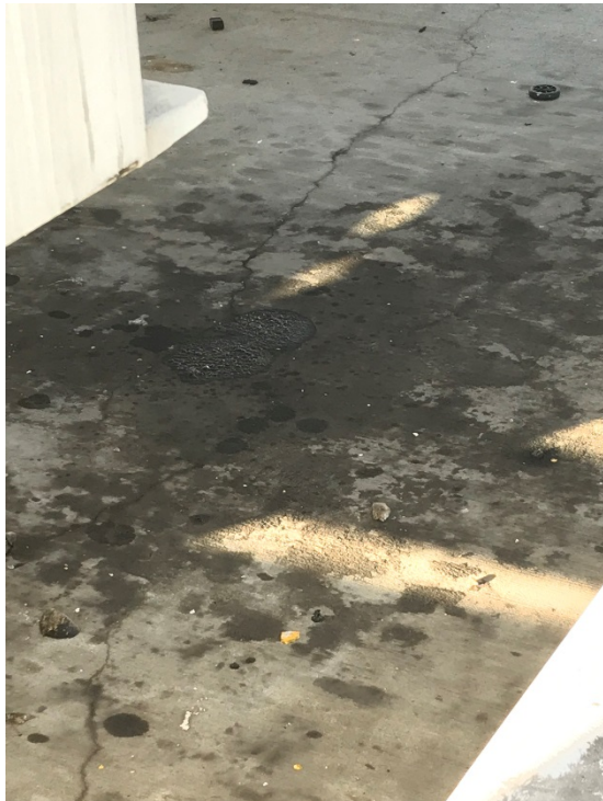
Photo 12 - Minor staining beneath passenger bridge lift system
