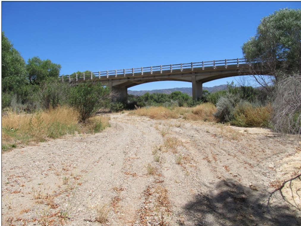
Photo 4. View of the south side of the Buckman Springs Road Bridge, looking north.
