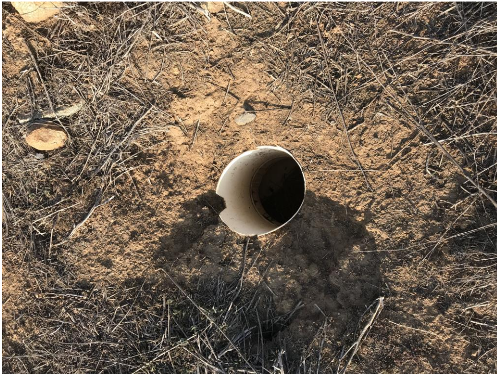
Vertical drain used to divert natural flow underground. (Lake Mathews Reserve)
